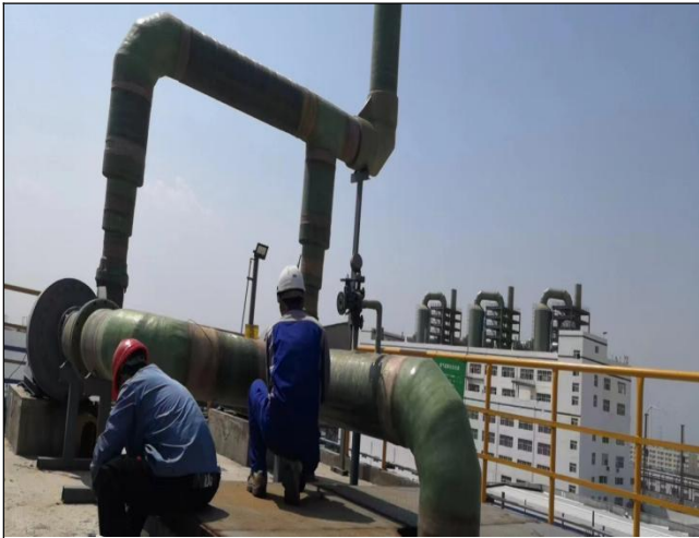
3 号碱吸收废气排气筒
