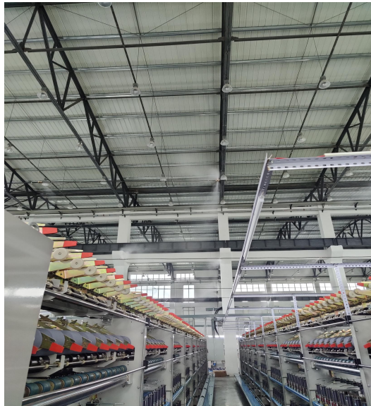
车间内水雾喷淋
