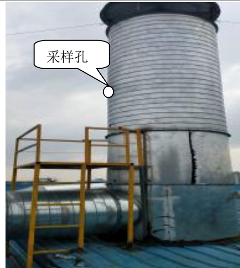
涂装工序+喷塑工序排气筒
