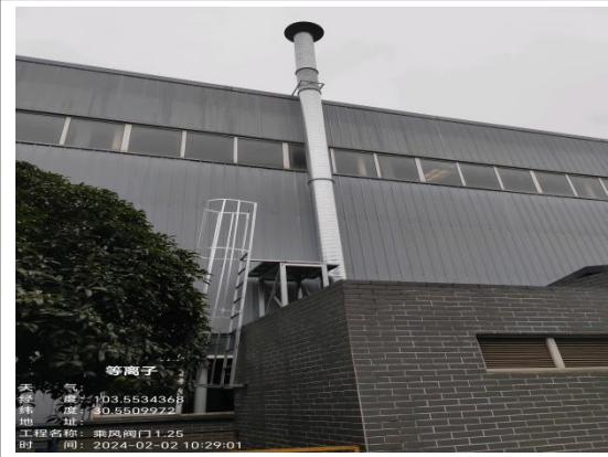
DA005 等离子切割废气排气筒
