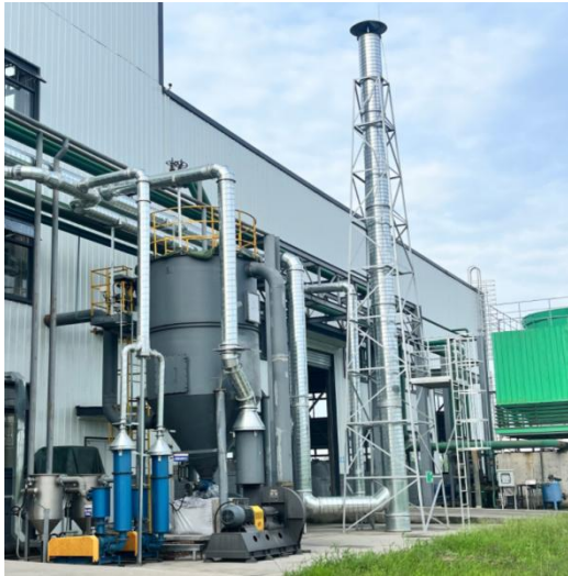
覆膜布袋除尘器+20 号废气排气筒 DA012
